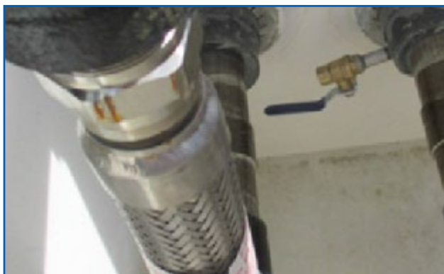
Flex Pipe Fitting in Dispenser Sump
