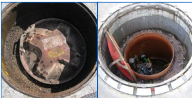
Sump Cover Closed
