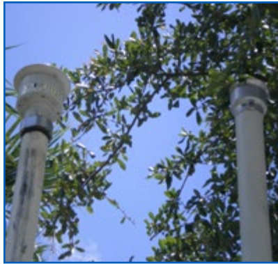
Vent Lines with Valves Installed
