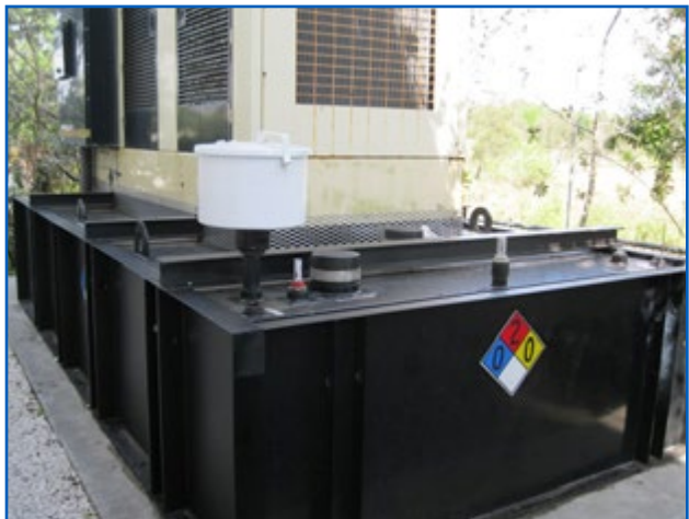
Sub-base DW-Emergency Generator AST
