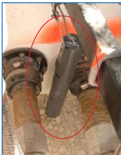
Sensor Placed Near Sump Bottom
