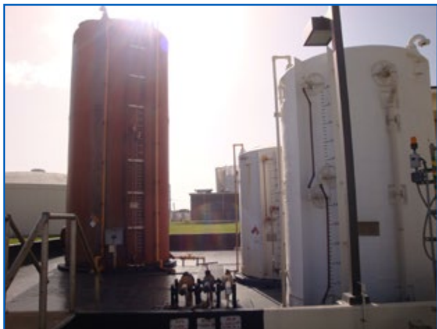
Vertical SW-AST within Secondary Containment
