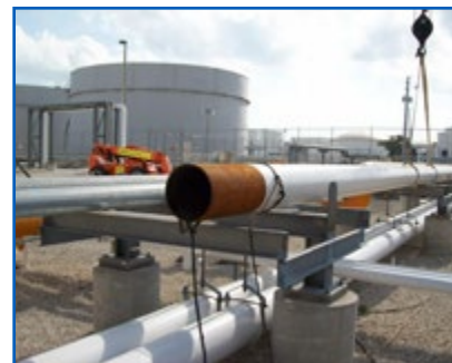
Bulk Product Piping
