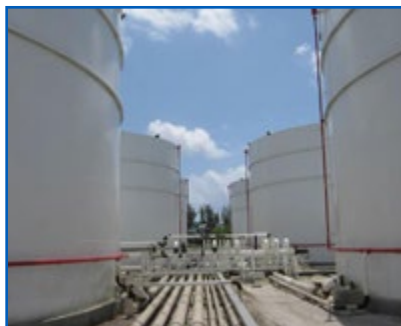
Piping for Field Erected AST
