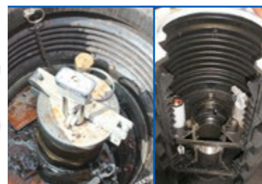
Release Valve in Spill Bucket
