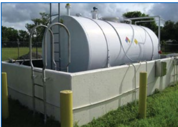
Single-walled Steel AST Inside Concrete Secondary Containment
