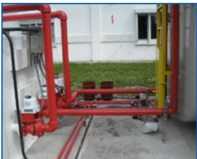
Piping for Shop Fabricated AST
