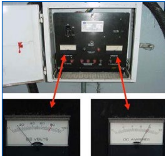
Impressed Current Rectifier with Voltmeter and Ammeter
