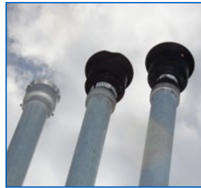
Vent Valves Extend 12 feet Above Grade
