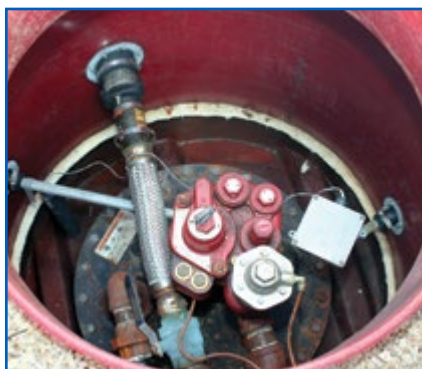
Piping, Pump and LLD inside Sump
