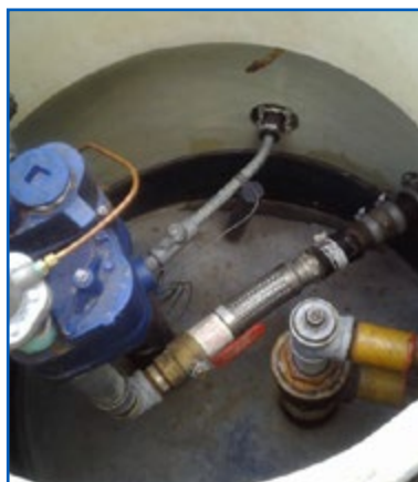
Flex Pipe Fitting in Pump/Piping Sump
