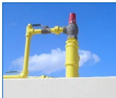
Anti-siphon Valve with Isolation Ball Valve
