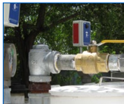
Anti-siphon with Isolation Ball Valve
